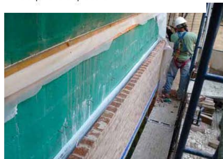
Installation of a rainscreen system. "The rainscreen approach operates on the assumption that water will inevitably find a way into a wall," says building envelope expert Bradley Carmichael.
